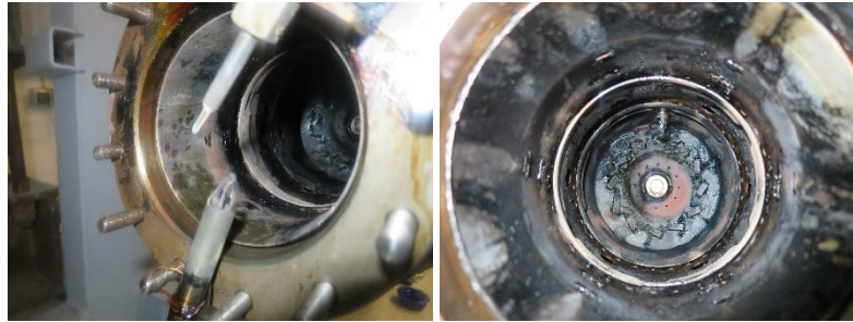
Fig. 10 Tar deposits on the fire tube's interior walls
