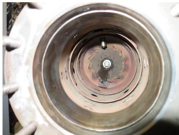
Fig. 2 The fire tube interior
